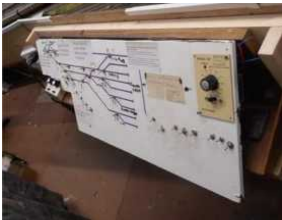
Above is a picture of the old Shunting Yard panel that has been in place for many years.
