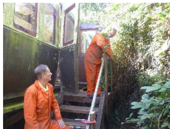
(John Waters (above) and Ronnie Wainhouse working on the new entrance steps to the Tintern coach.)
