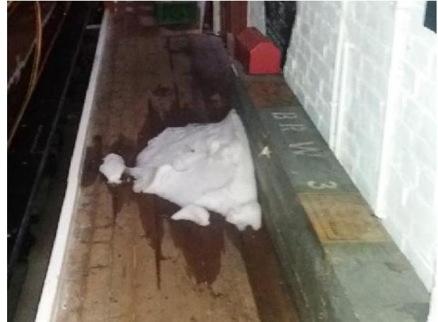
Snow lying in the floor by the extension Fire Door.
